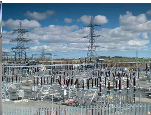
รูป OUTDOOR SUBSTATION
