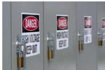
Indoor Switch Gear
