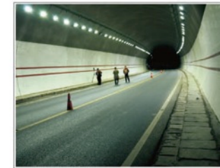
LED Tunnel Light
